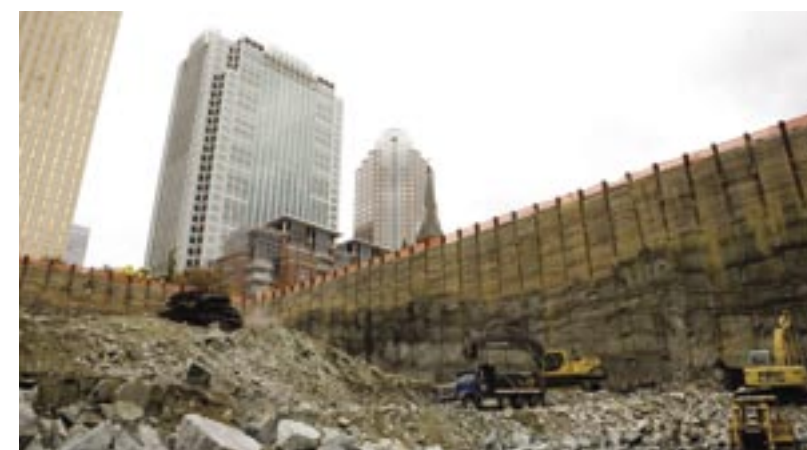
Crews work to remove the granite foundation of the new Wachovia office tower.
